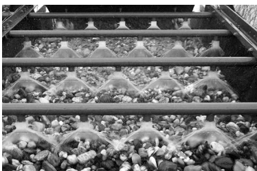
High pressure spraybars with plastic nozzles
