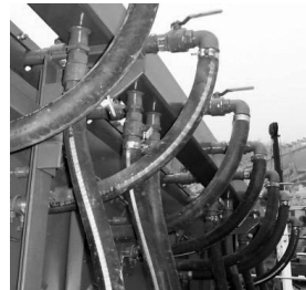
Integrated manifold with ball valve and high pressure rubber hosing
